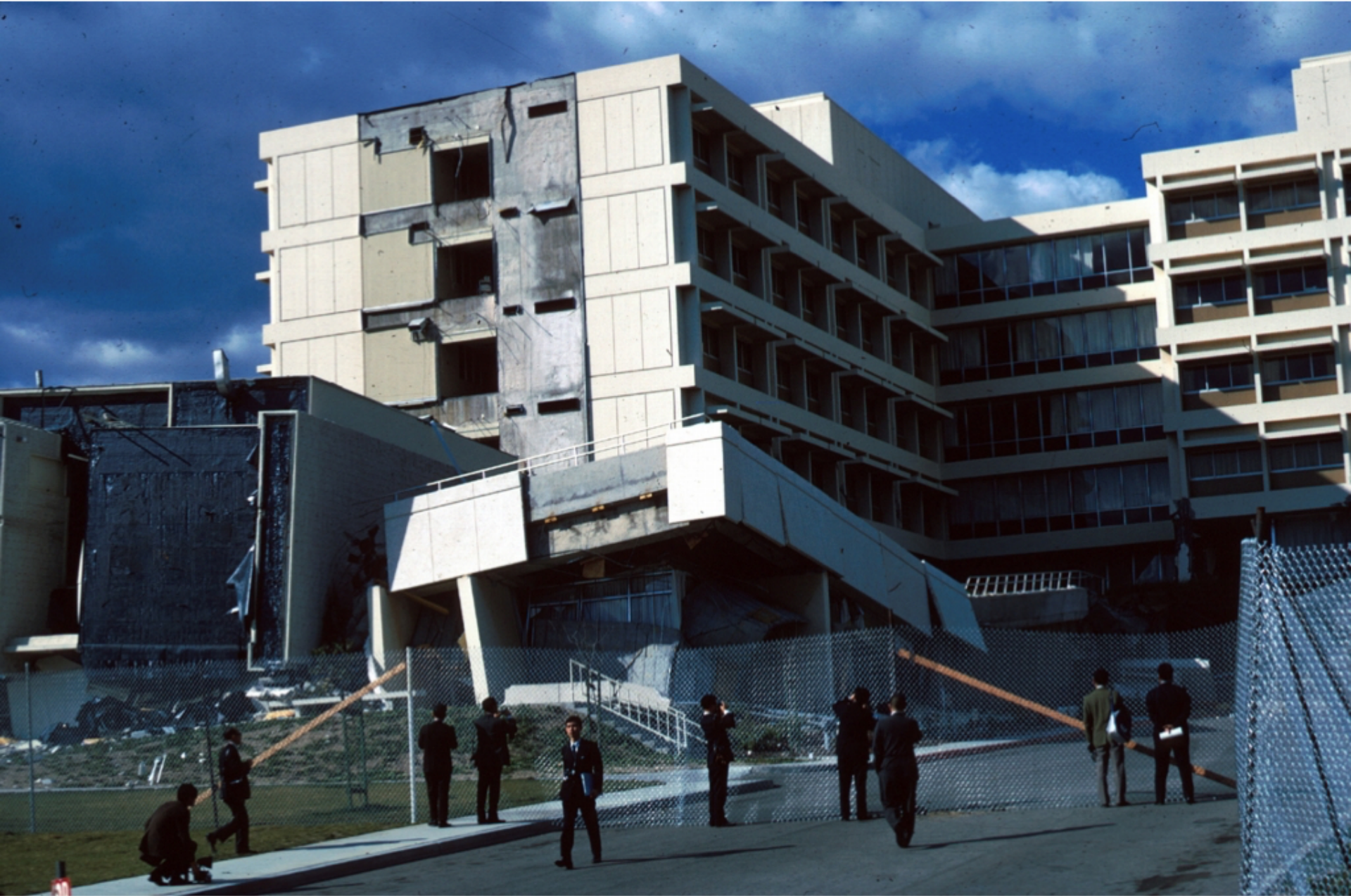
Olive View Memorial Hospital, Sylmar, California Destroyed with lives lost in the San Fernando Earthquake, 1971
