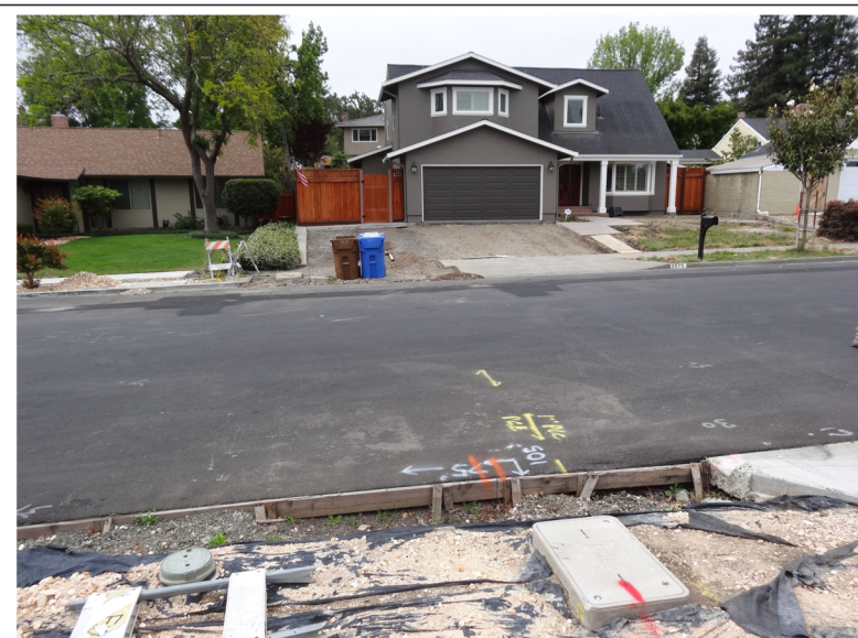
Students were subsequently introduced to the South Napa earthquake of 24 August 2014, which caused $400M in damage even though it was just a M6 event. Buried utility lines were extensively damaged.
